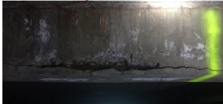
Fig. 2. Longitudinal cracks in prefabricated reinforced concrete girders, opening width a_T = 5 \dots 20 mm at level +11,200 (4th floor)
