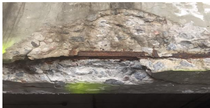
Fig. 1. Soaking of the girders at level +11,200 (4th floor), on the axis «1» in the axes «Д-Е», corrosion of the working reinforcement, peeling of the protective layer of concrete
